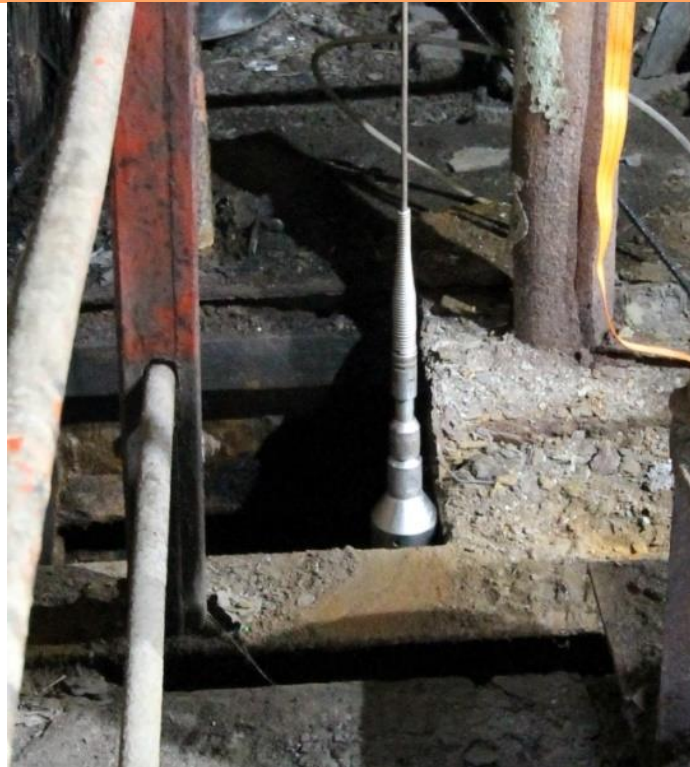
Figure 2 – Survey Datum (Probe datum is widest point of shoulder)
